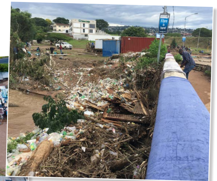
The Quarry Road West bridge which was blocked with alien vegetation, indigenous vegetation and solid waste (Source: Cathy Sutherland, 12 April 2024)
